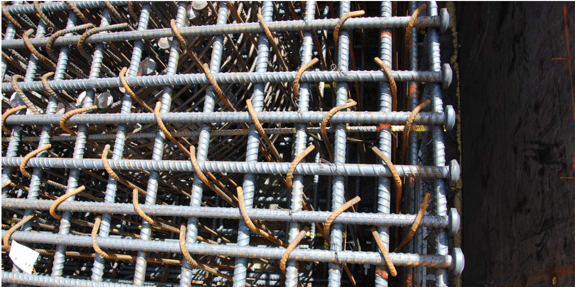
Picture (plan view) of headed bars in a foundation, meeting the general requirements outlined above
